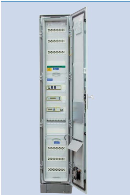
IT system distribution cabinet TR-VITC
